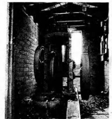
HIGH AND DRY —This old, rusted pump in the well house was the first used to pump water for the Brandeis ranch. The well has been abandoned.
